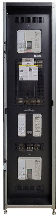
Maintenance bypass (door removed)
