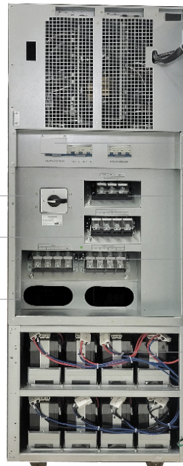
E91-40K front view (door & panels removed)
